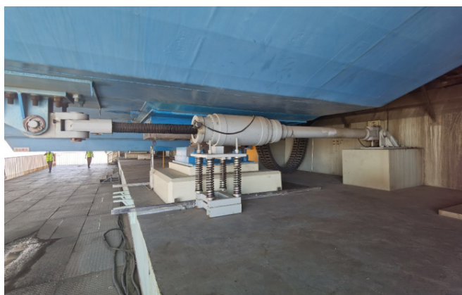
Figure 3-5-8 Large-tonnage Eddy Current Damper Application Case - Jiangyin Yangtze River Bridge
